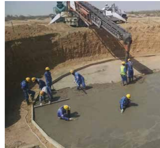
Construction of the now operational Metro Wind power plant, Sindh Province, Pakistan
