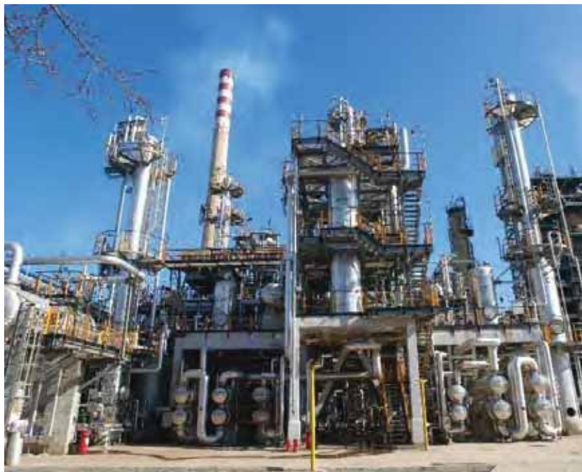
Sisak is one of INA's two main refineries and is located near Zagreb. ICF-DP funds were used to help complete Phase I of the plant's infrastructure modernisation plan
